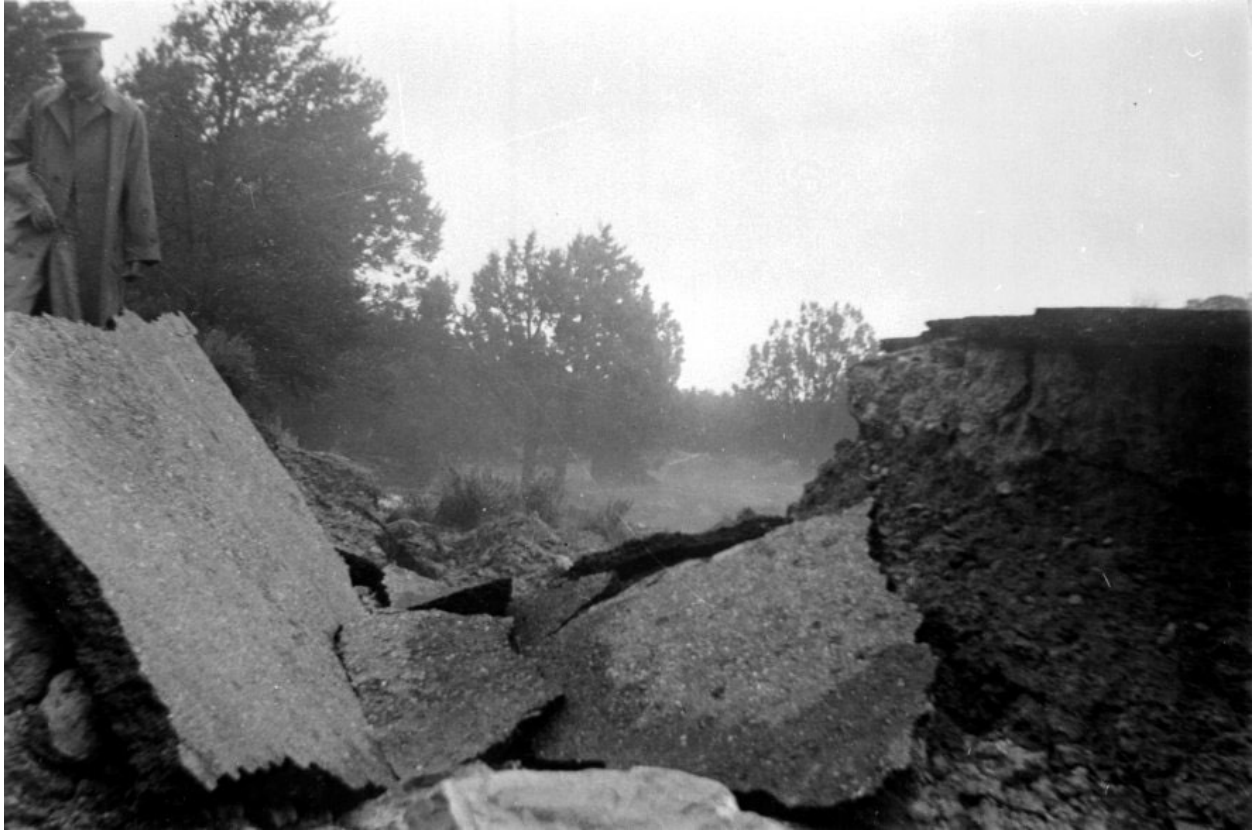
#12770: A rain and hailstorm damaged the East Rim Drive, in July 1946.
