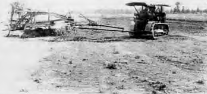
Using road machinery loaned by the Park Service, Emery Kolb prepares his landing strip near the Lauzon homestead.
