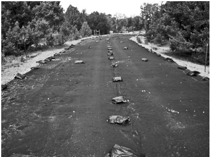
Synthetic fabric is held down by sand bags to keep radioactive dust and other contaminants contained.
