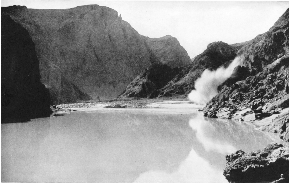
Blasting in the Inner Gorge at the site of the bridge, 1921. Photograph by the Kolb Brothers
